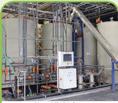
Neue Mischanlage New mixing equipment
